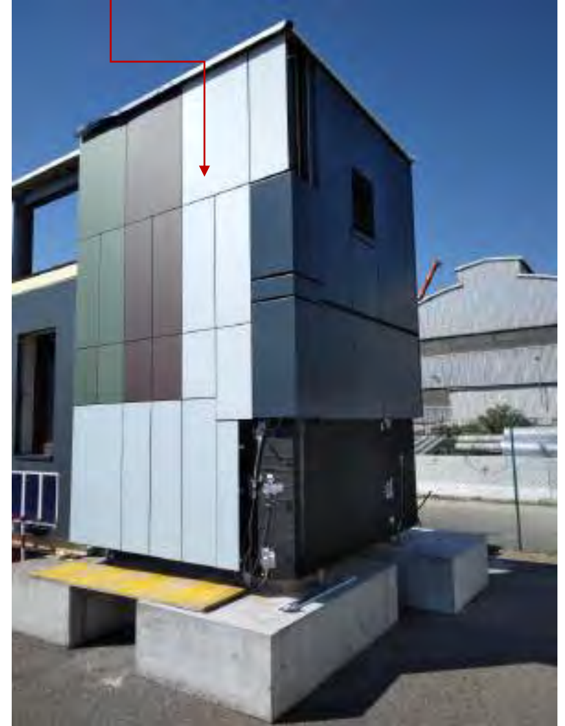
BIPV installed on-site (due to fragility)
